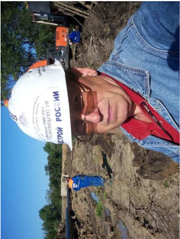
The island of Sakhalin. Construction of «Unit Kirinskoye gas and field project «Sakhalin-III» Chief welder of FSUE «GOOSSEN «Dalspetsstroy when Spetsstroy of Russia» Anatoly Ivanovich Brëkhov 11.03–29.04.2012 year.
